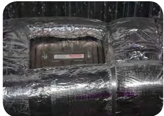
Duct access must be insulated (not bare) Shown is a typical factory door
