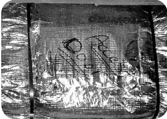
Insulation cover must be removable Tape is not sufficient to hold insulation
