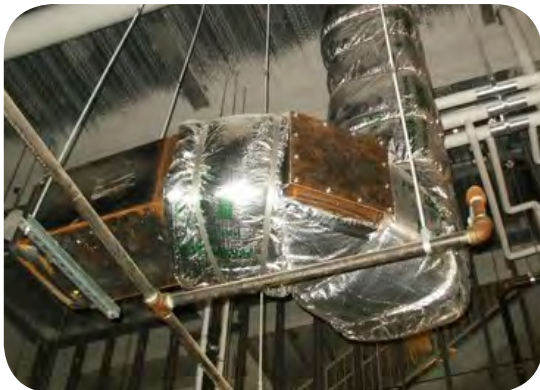
Avoid flanges taller than insulation This typical door is tough to insulate
