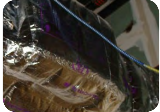
Tape is not sufficient to hold insulation Use weld-on pins to attach insulation
