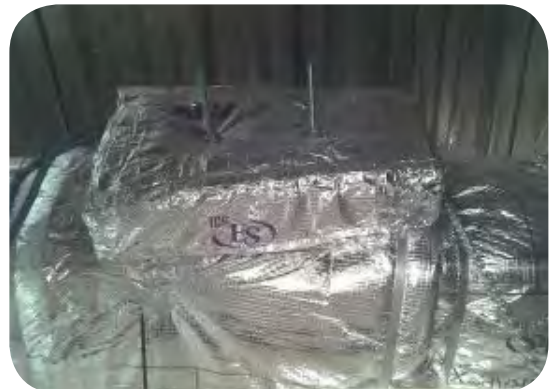
Code requires door be insulated This door only has a clearance shield
